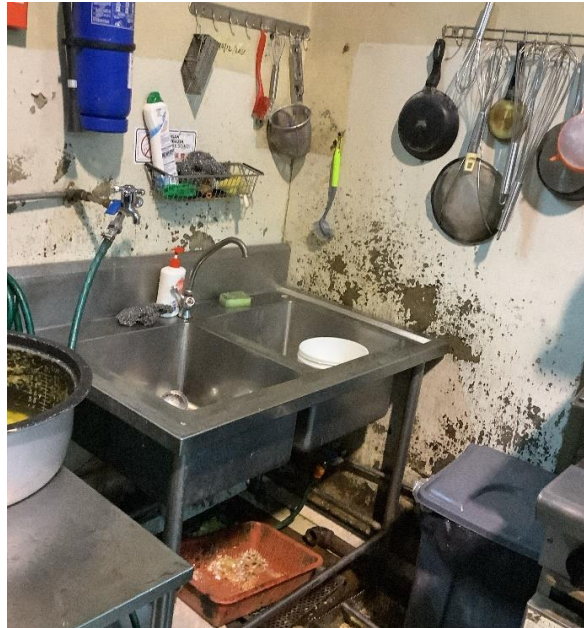
Peeling wall paint and cracked discoloured floor tiles (Photo by SFA)
