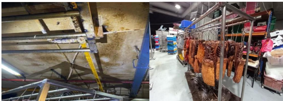
Left: Dirty ceiling observed during inspection Right: Roasted meat stored outside the premises (Photos: SFA)
