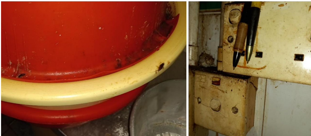
Hygiene lapses detected include the presence of vermin and poor cleanliness of the switches at the premises (Photo: SFA)
